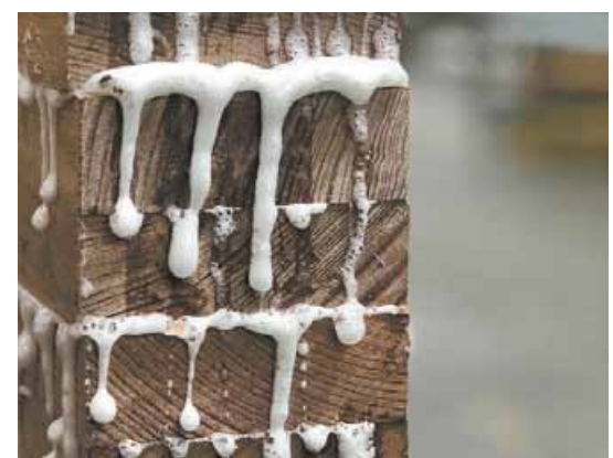
■ Glue runs on ends of beams from factory.
